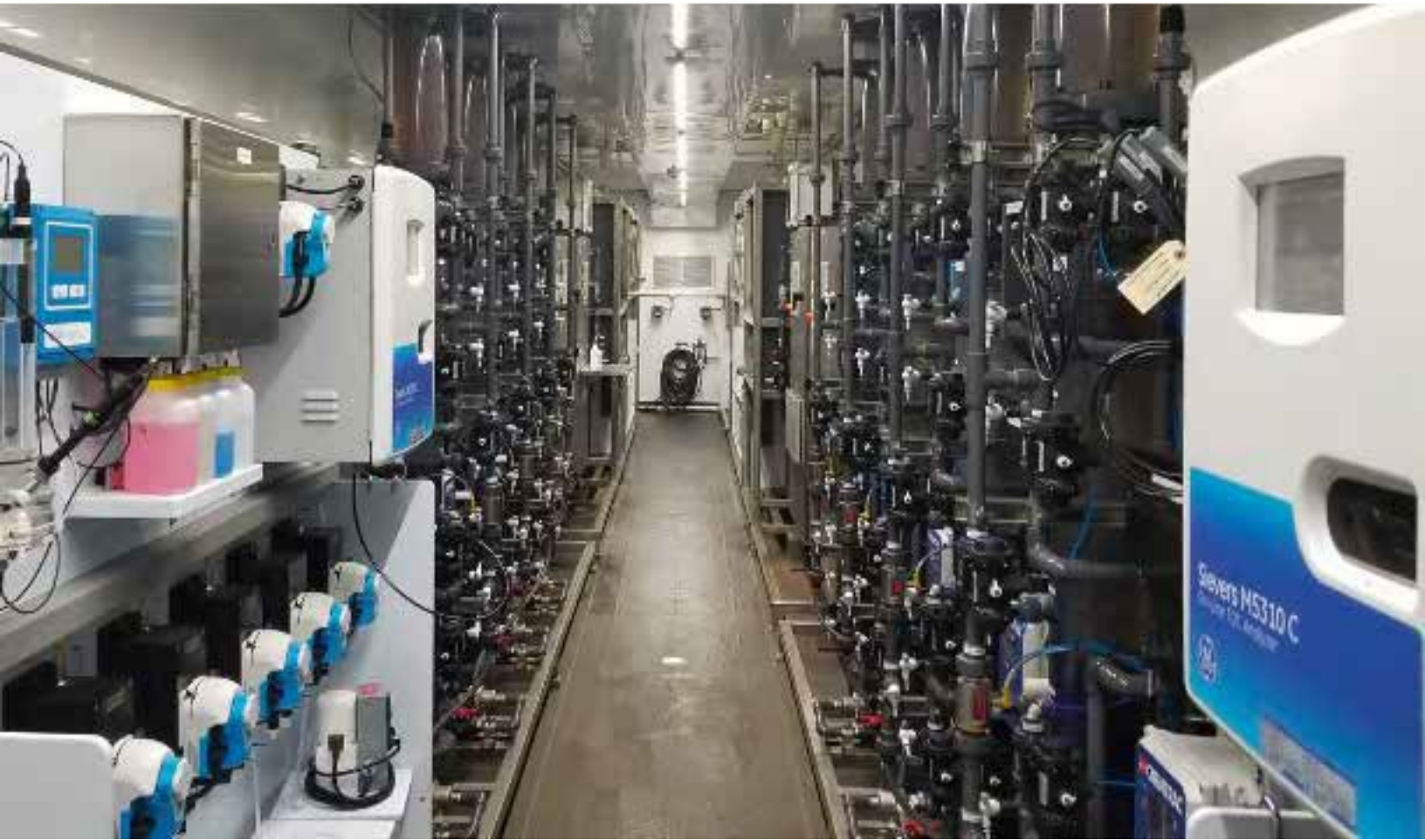
BWW'S MOBILE PILOT PLANT TESTS WATER PROCESS TREATMENT ALTERNATIVES.
