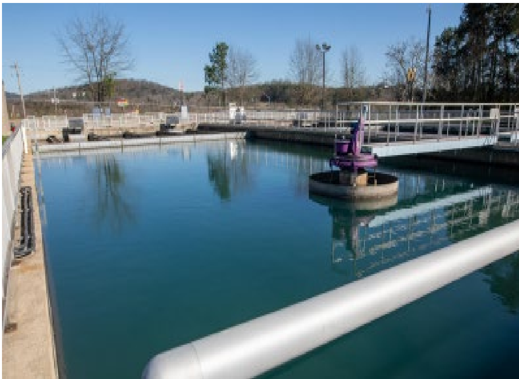
CARSON FILTER PLANT
